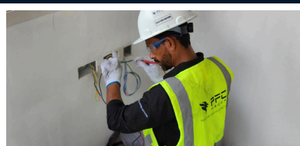
Electrical DB Installation- MEERAS
