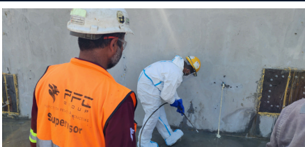
Chemical Injection Works- AD Ports
